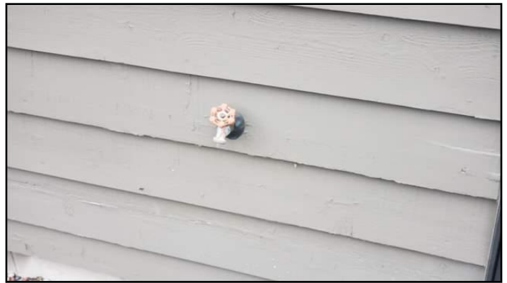
Missing Backflow Prevention
