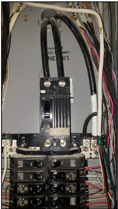
200 Main Power Service Feed Inspected
