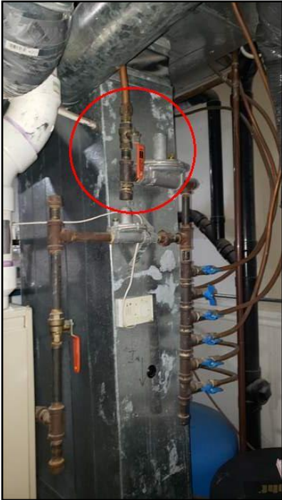
Main Gas Shut Off
