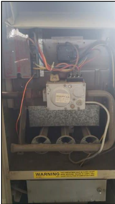
Garage Furnace Inspected
