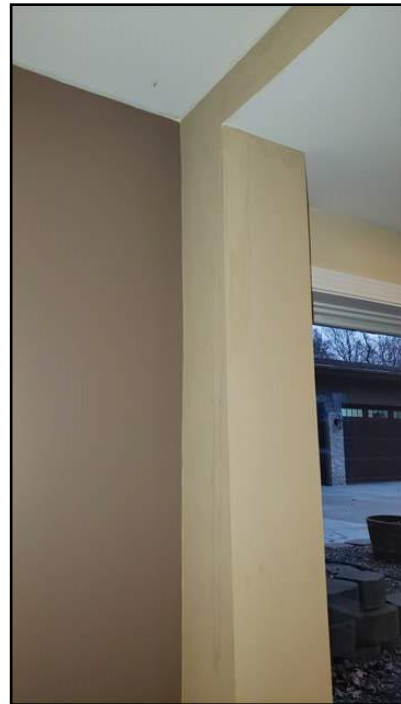
Sign Of Moisture
