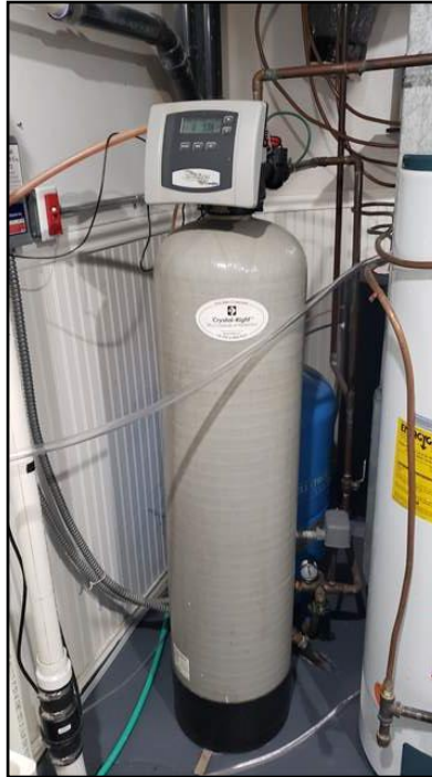
Water Softener Noted
