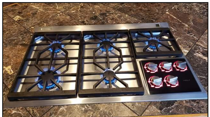
Range Burners Ran and Functioning
