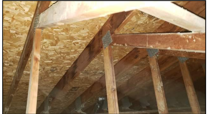
Sign Of Moisture
