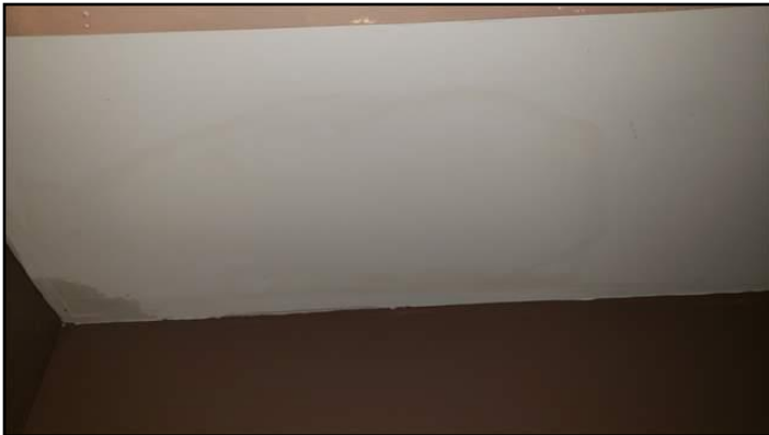
Sign Of Moisture
