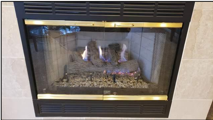
Gas Fireplace Ran and Functioning
