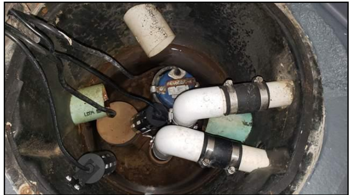
Sump Pump and Backup Pump Tested
