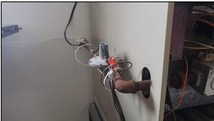
Potential Leak @ Gas Line
