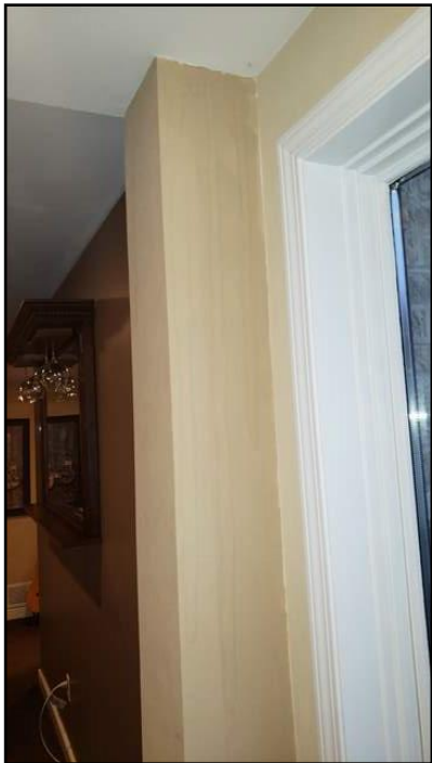
Sign Of Moisture
