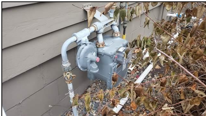
Potential Leak @ Gas Line
