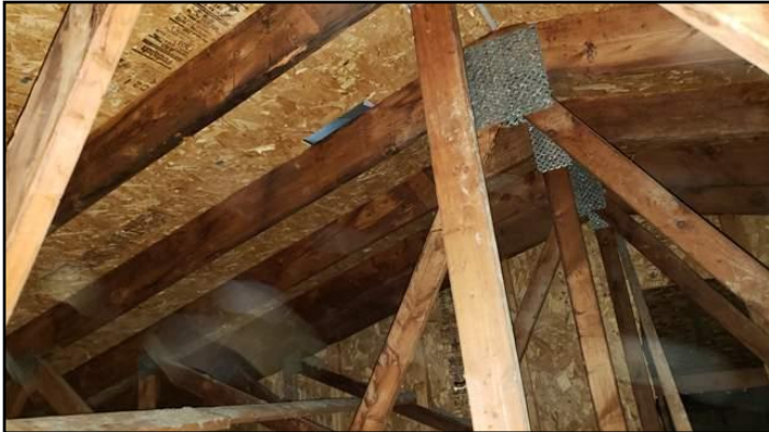
Sign Of Moisture
