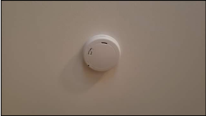
Smoke/CO Detectors Tested
