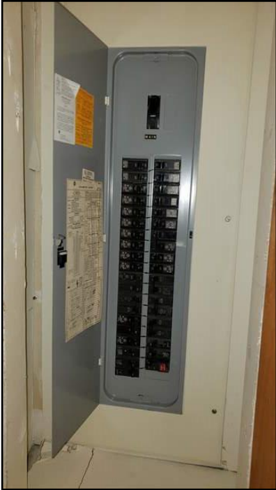
Main Panel Inspected
