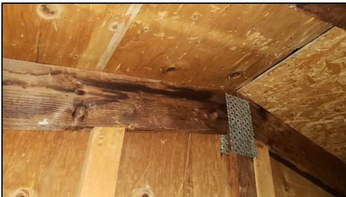
Sign Of Moisture
