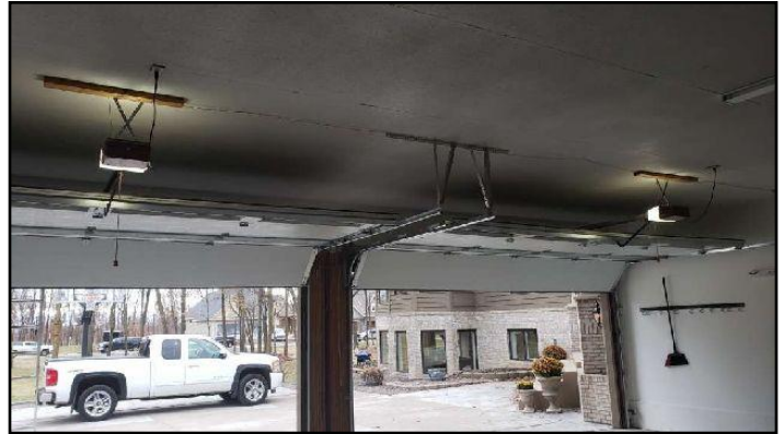
Garage Doors and Sensors Ran and Functioning
