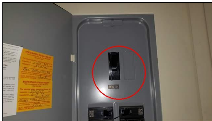
Main Shut Off
