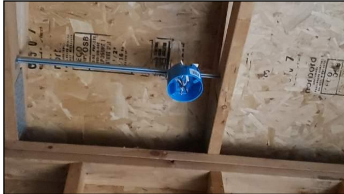
Missing Cover Plate
