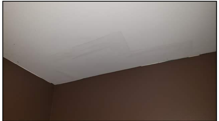
Sign Of Moisture
