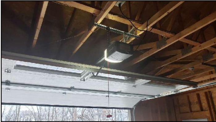
Garage Door and Sensors Ran and Functioning
