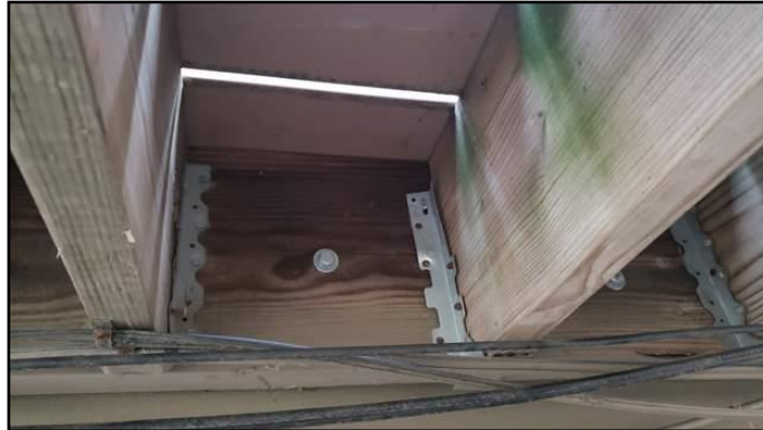
Missing Flashing @ Ledgerboard
