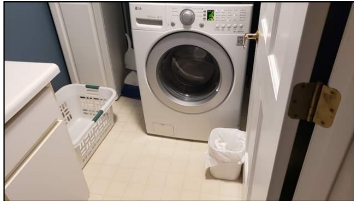
Missing Drip Pan
