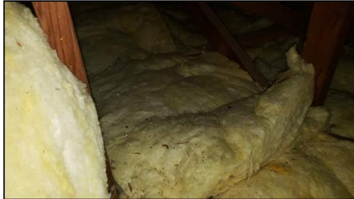
Glass Fiber Insulation Noted
