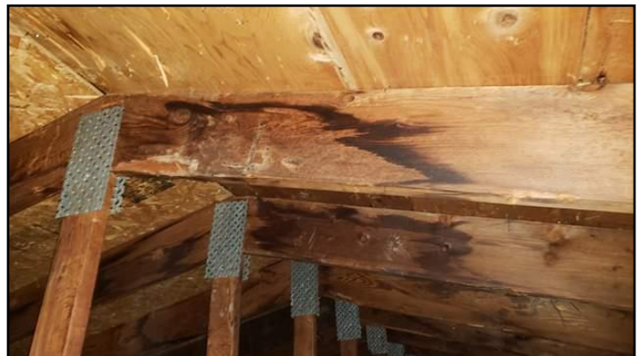
Sign Of Moisture
