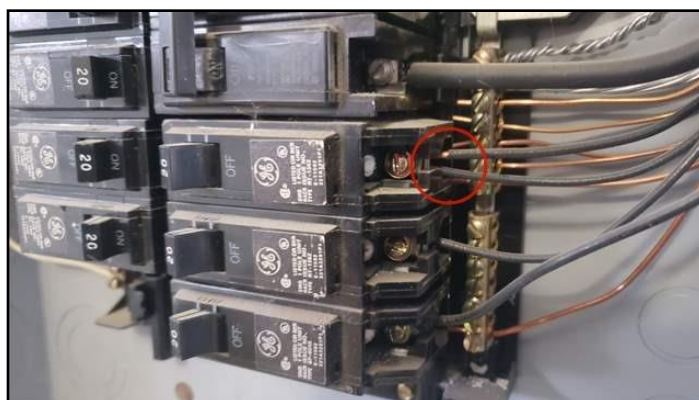
Double Tapped Breaker
