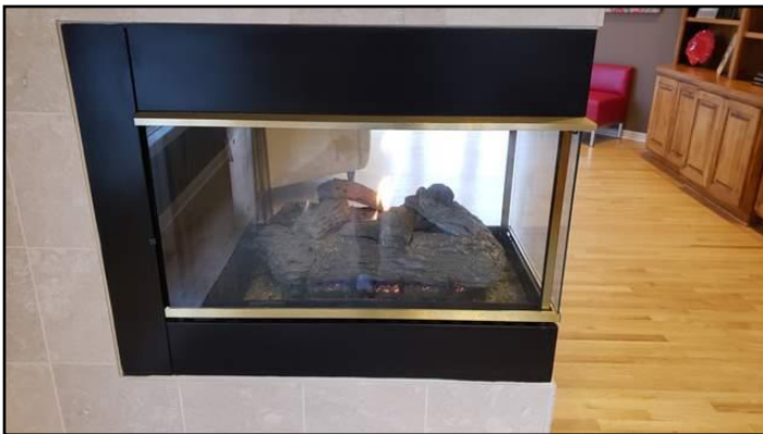
Gas Fireplace Ran and Functioning
