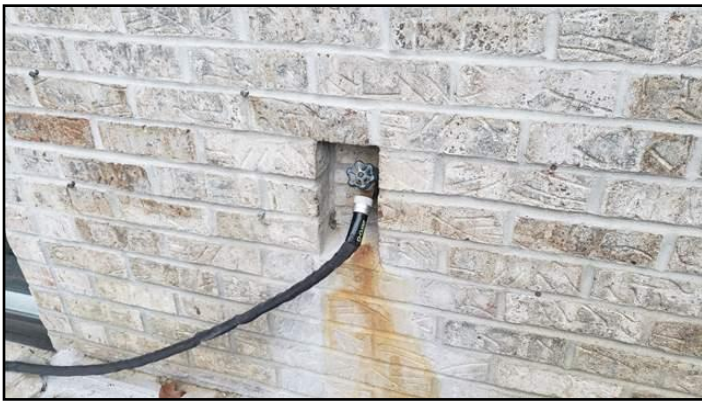
Missing Backflow Prevention
