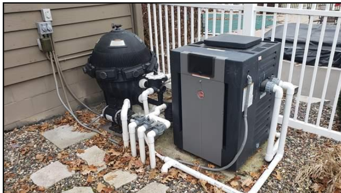
Pool Equipment Not Inspected
